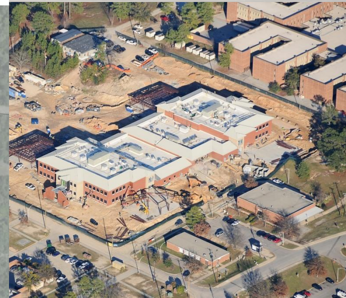
Construction of a Basic Training Center and Quad Dining Facility at Fort Jackson
