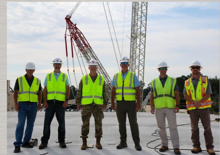
USACE personnel during the construction of a new parking garage at the Columbia Dom VA Medical Center
