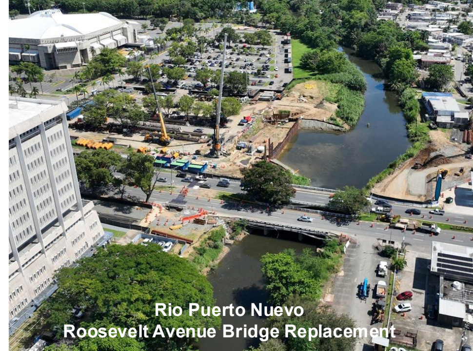
Rio de La Plata Dorado Bridge Channel Widening and Scour Protection, and ACBM Toe Key Construction
